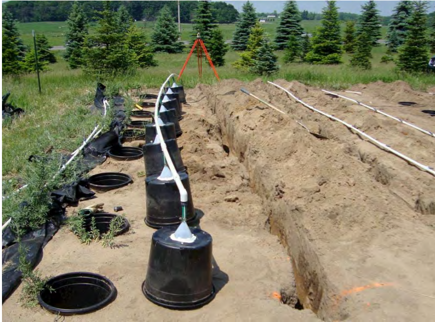
Figure 2. Installation of leachate collection system. Each row of 8 trees drains to a single line. Run-off from each line was continually measured by tipping bucket rain gauges and an automated datalogger.
