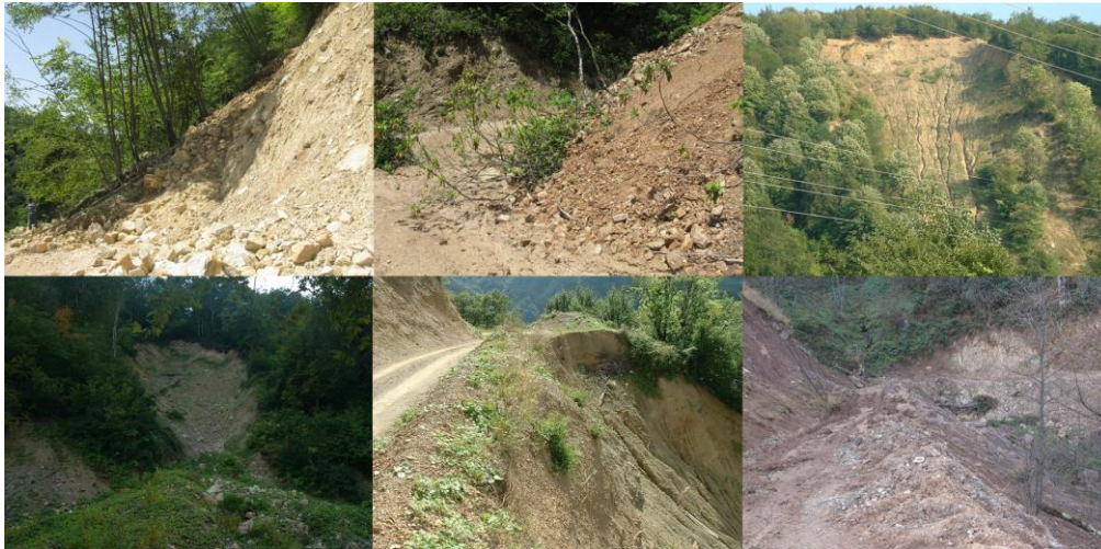
Figure 1. Forest roads damaged by landslides
