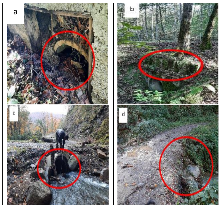
Figure 7. Various failures in pipes across the investigated roads, a, b, c) Intel cracking of pips, d) culvert with the destroyed outlet
