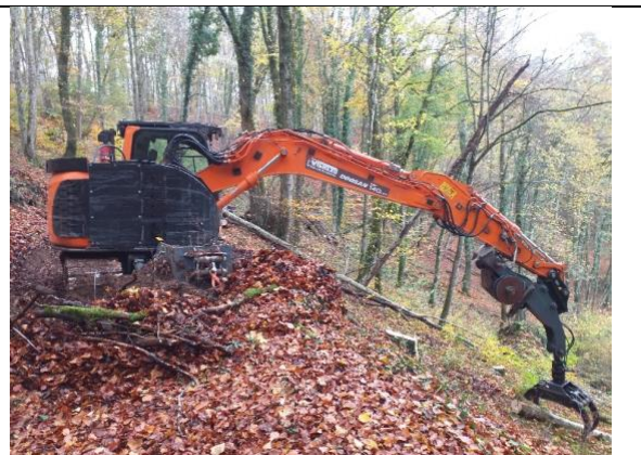
Figure 6: When the grapple is used, the multifunction hub is stuck under the boom
