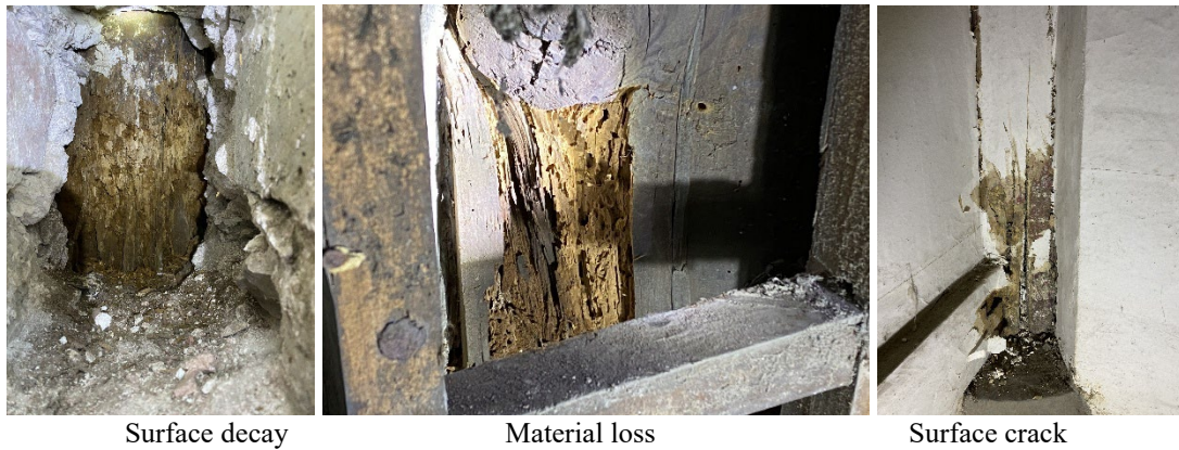
Figure 3 —External defects of the wall wood columns
