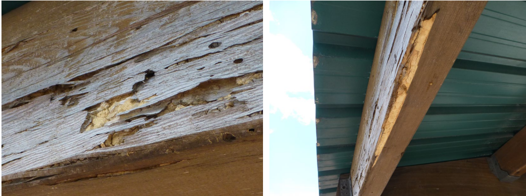
Figures 1 and 2—Damages by Hylotrupes bajulus in glulam beams.
