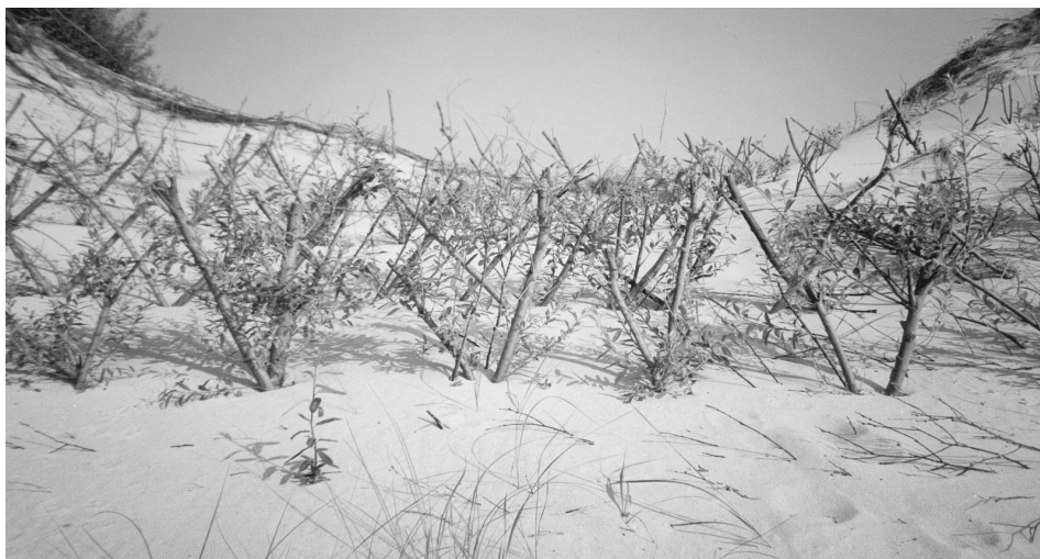
Fig. 2. Openwork live protections of willow stakes for restoration of a destroyed foredune site in a kettlehole.
